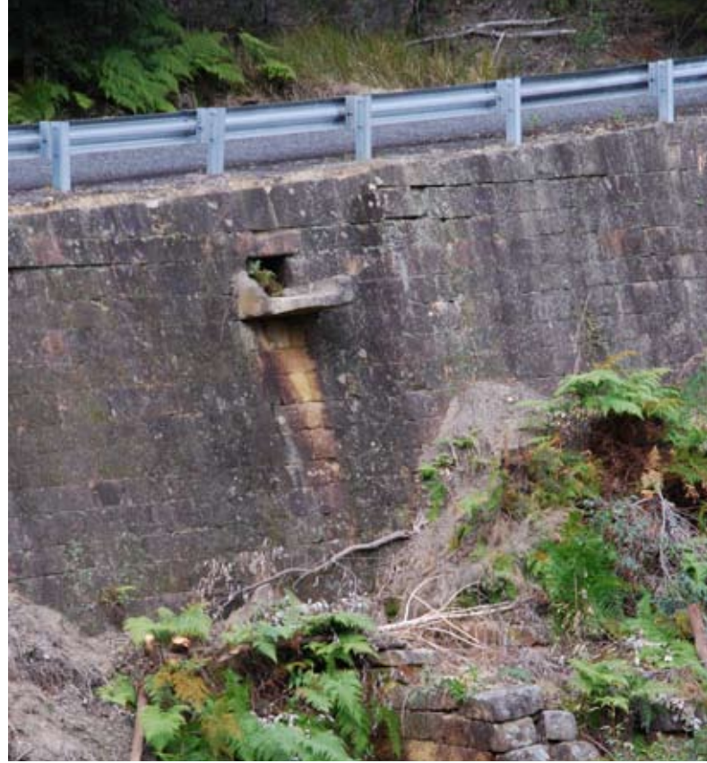
The new section of the SHR listed Great North Road features several unique structures including the Ramsay's Leap culvert and stone wall (pictured), St Alban's Road ramp and the timber Thompson's Bridge.
